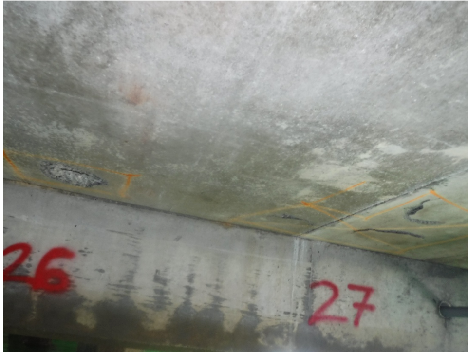
Photo 1: Typical Precast Plank Soffit Spalls at Pier 17
