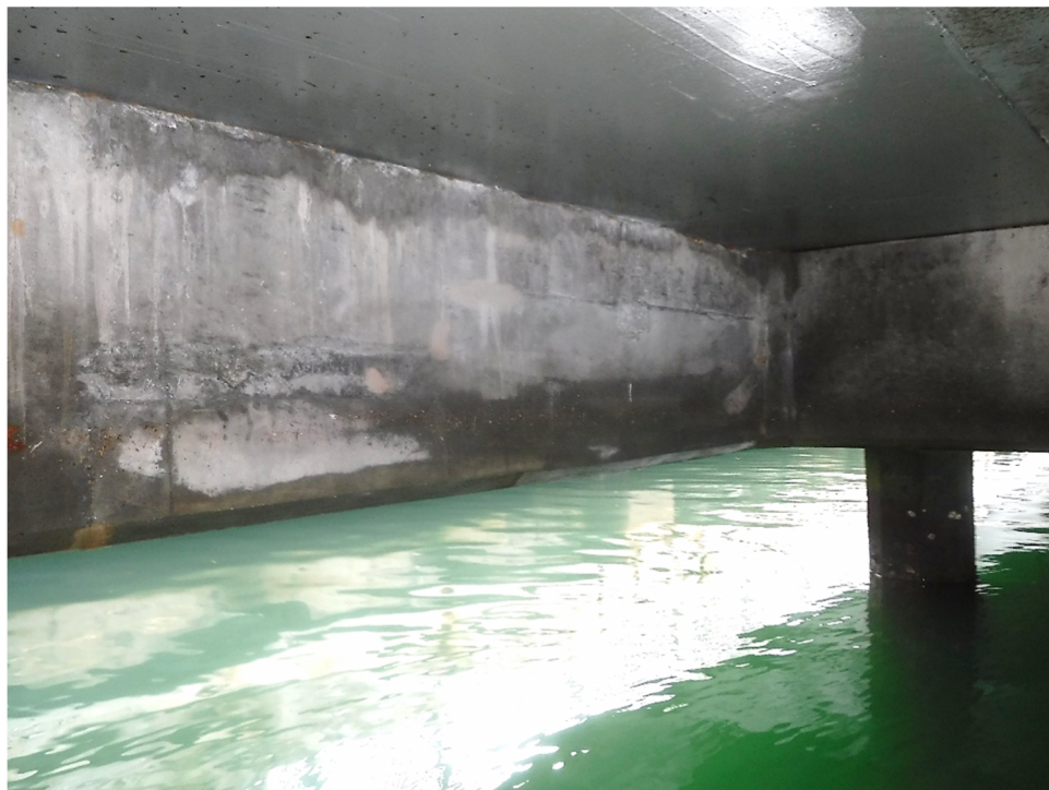
Photo 2: Typical Beam Spall at Pier 17
